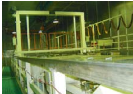
▲The Chemical/electrochemical Cleaning Equipment
