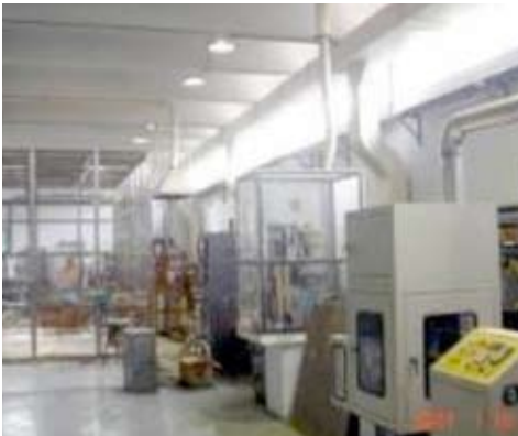
▲Before Cleanup of Room 110 in Building 021
