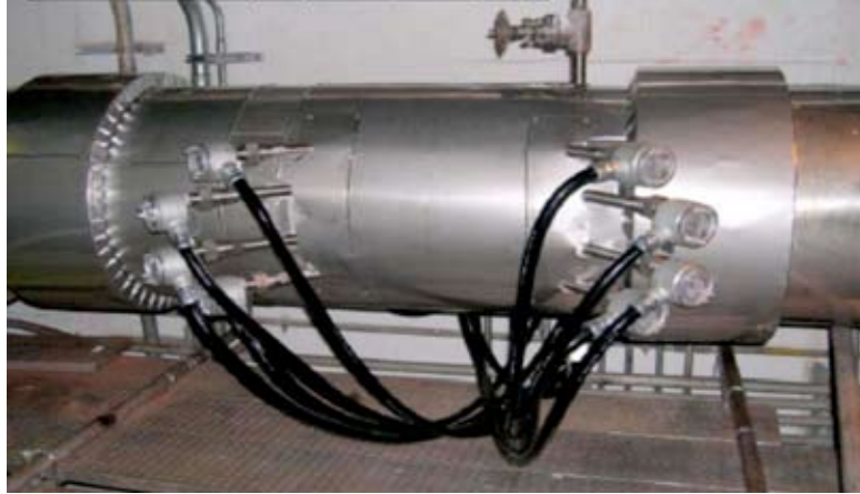
▲The UFM System (Caldon LEFM CheckPlus) Installed at Kuosheng NPP
